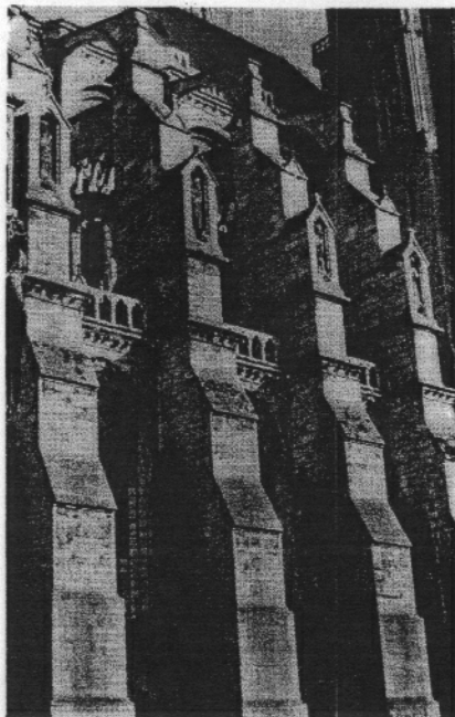
20 Chartres nave buttressing. Flying buttresses are almost hidden by the massive pier buttresses. Photo by J. Hart.
